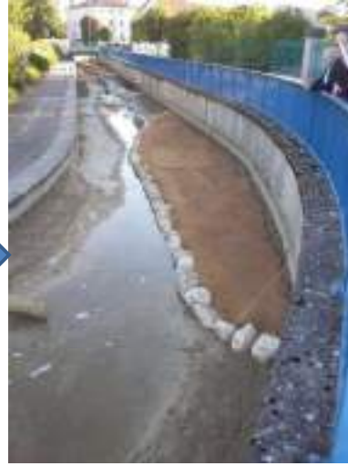
Picture 5: Riverbank filled with earth, covered with a geotextile membrane, girdled with stones in Fresnes-en-Woëvre (Sept. 2016)
